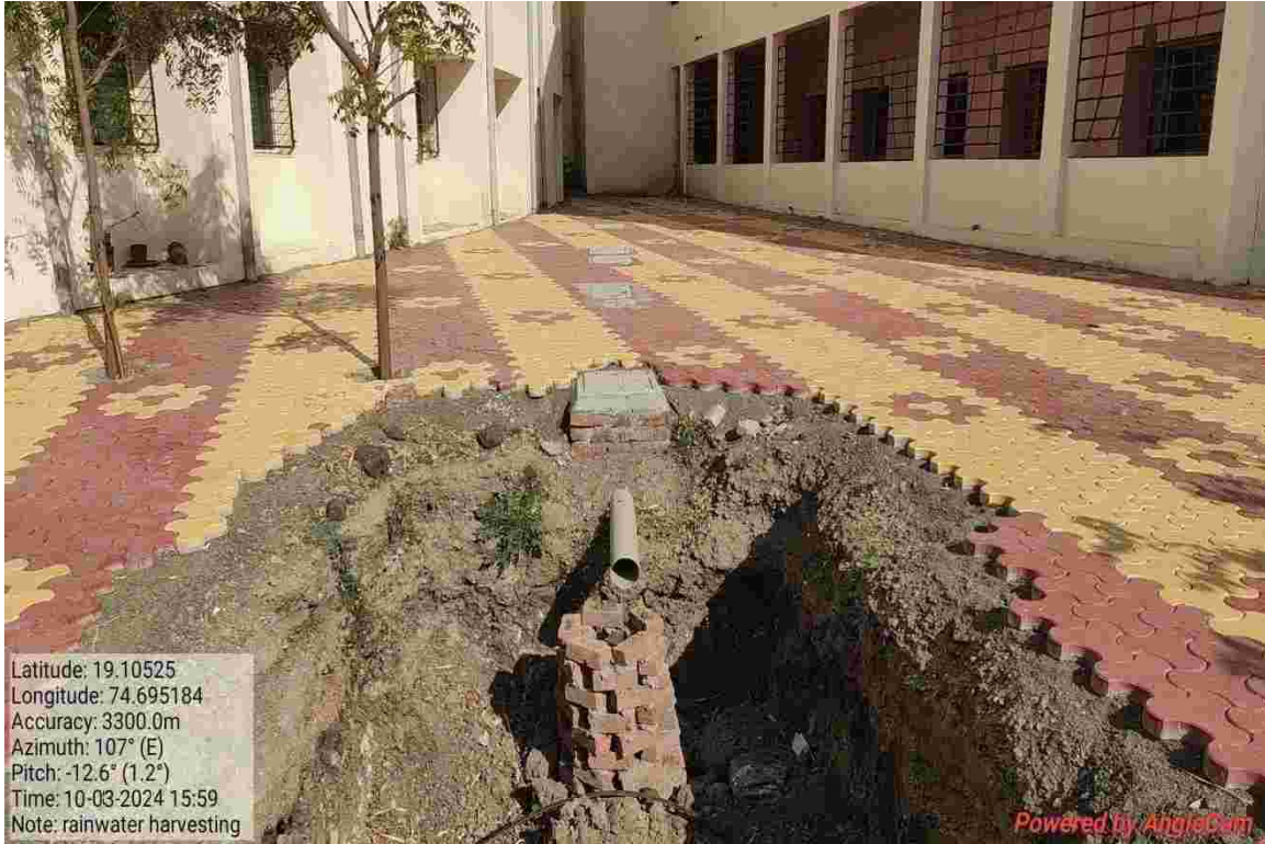
Ground Water Recharge Pit
